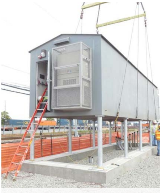
PATH Signal Bungalow Raised Elevation
