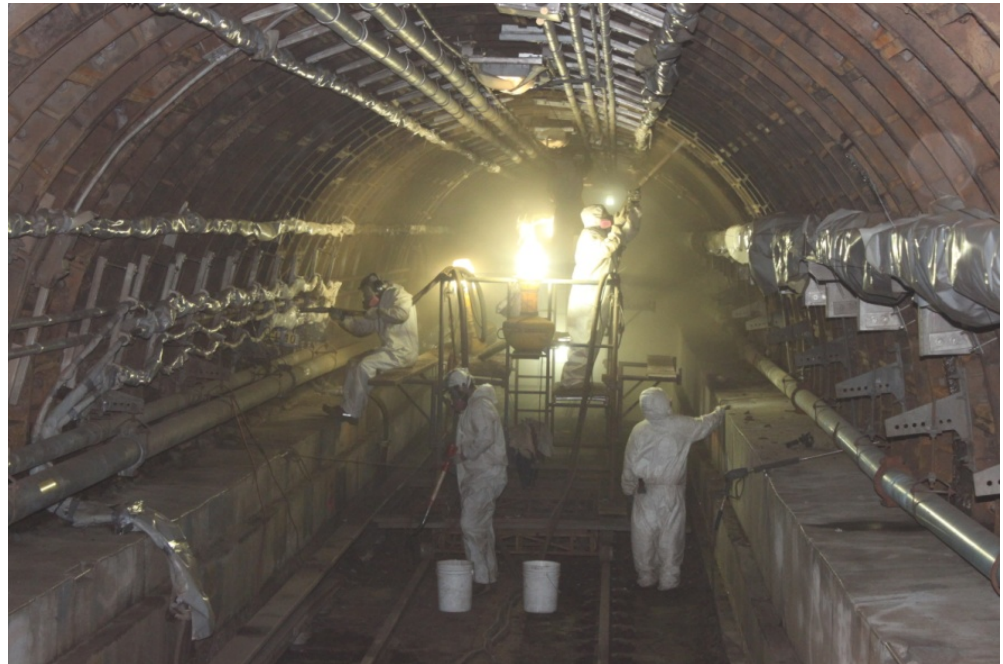
PATH Tunnel Desalination (Latent Damage)
